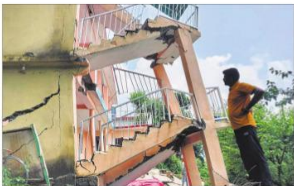
A damaged house in Dharampur subdivision of Mandi. JAI KUMAR
