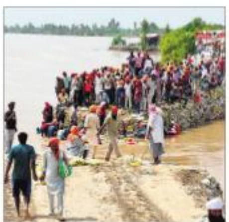
Work underway to plug a breach at Ghadam village in Tarn Taran.
